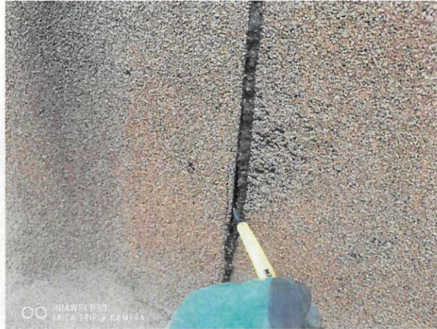
Figure 5 – Re-seal open seams
