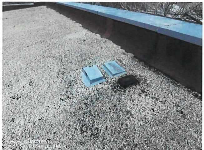
Figure 4 – Remove unused projections and seal, Roof B2
