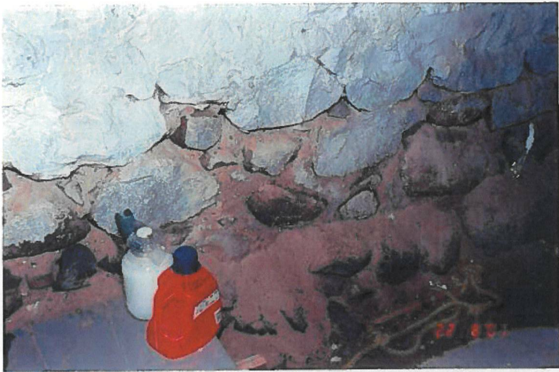
31. TYPICAL BASEMENT WALL SHOWING MORTAR FALLEN FROM JOINTS.
