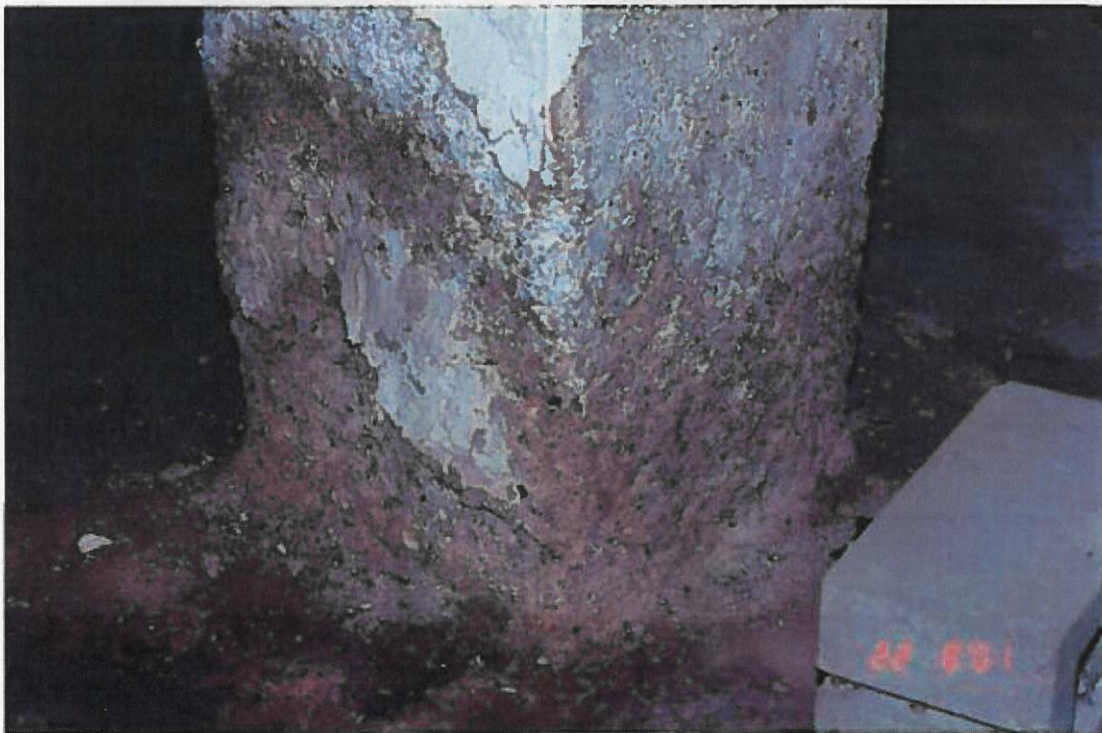
28. CONCRETE COLUMN DETERIORATION AT BASEMENT FLOOR UNDER "VAULT" - SOUTH END.
