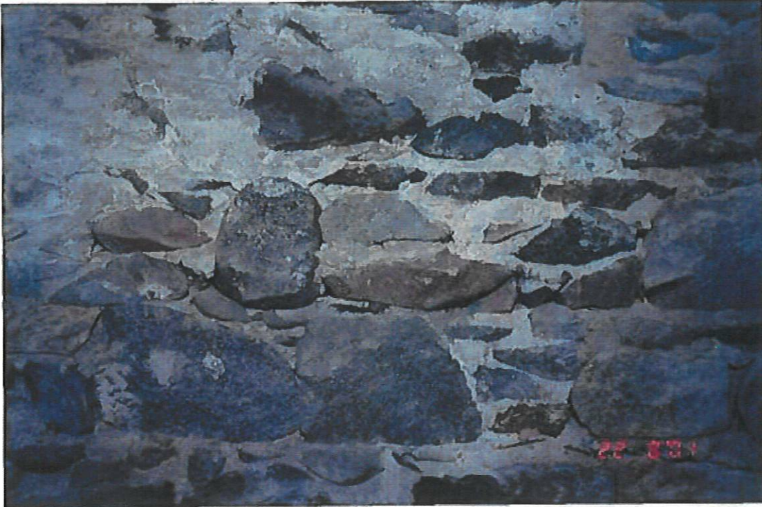
29. TYPICAL "FIELD STONE" BASEMENT WALL WITH DETERIORATED MORTAR JOINTS.
