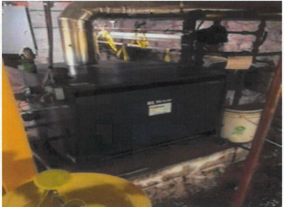
New Piping, Ducting and Boiler
